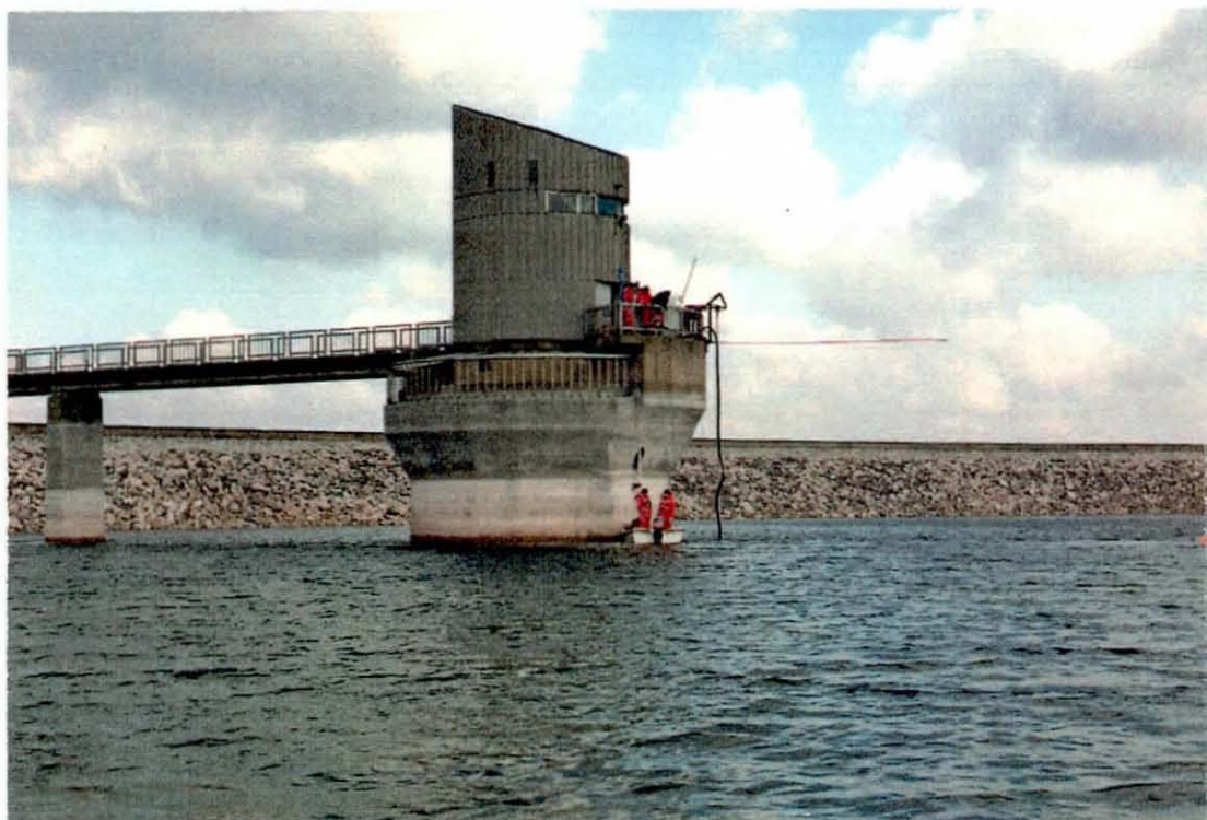
Fig.5.3/2 Foremark Draw Tower, outer working platform with free standing array support and hydrophone pole.
