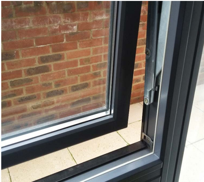
FIGURE 2. RESTRICTED WINDOW OPENING THRESHOLD, FLAT A LIVING ROOM
