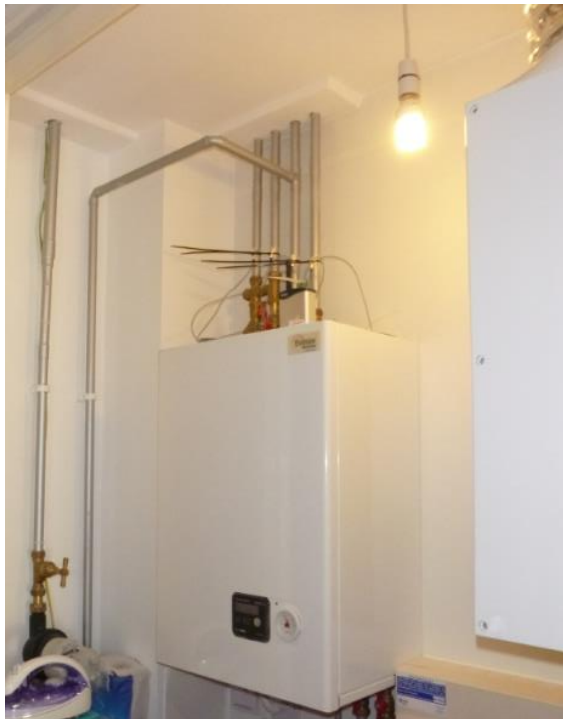
FIGURE 5. HIU - SHOWING UNINSULATED HEATING SYSTEM PIPES AND MVHR UNIT IN SHARED SERVICES CUPBOARD (FLAT C)
