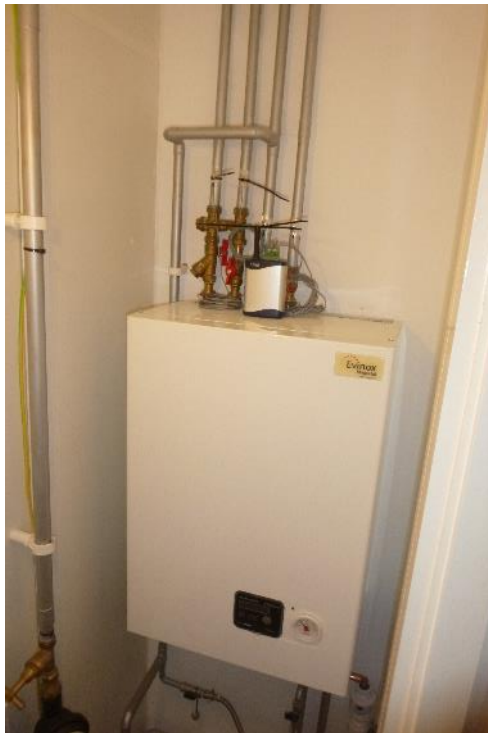
FIGURE 4. HIU - SHOWING UNINSULATED HEATING SYSTEM PIPES (FLAT B)
