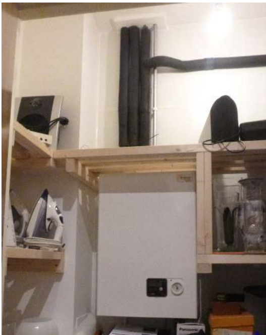
FIGURE 3. HIU SHOWING INSULATED HEATING SYSTEM PIPES (FLAT A)
