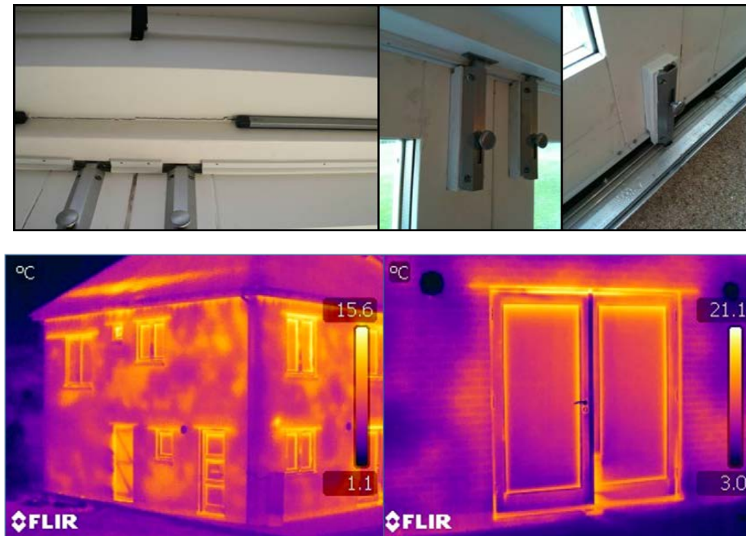
Figure 6 – Observational evidence of poor quality installation and of uneven cavity wall insulation.
