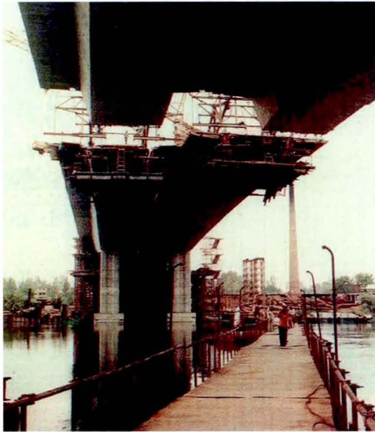
Figure 3.23: Using stationary system to construct one of the cantilevers ends (The Arab Contractors, 1991)
