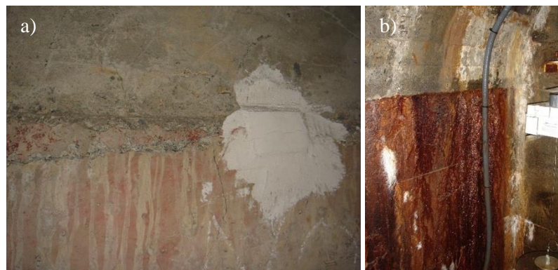
Figure 3. a) Cracking and b) ochre shading precipitate in the gallery.
