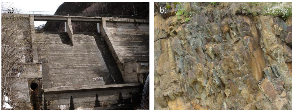
Figure 1. a) General view of the downstream face in 2005 and b) slates found near the dam.
