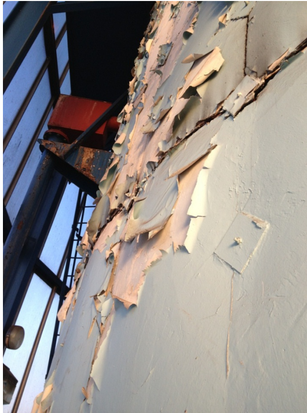
Figure 20. Superficial damage to the accumulator's plaster coating
