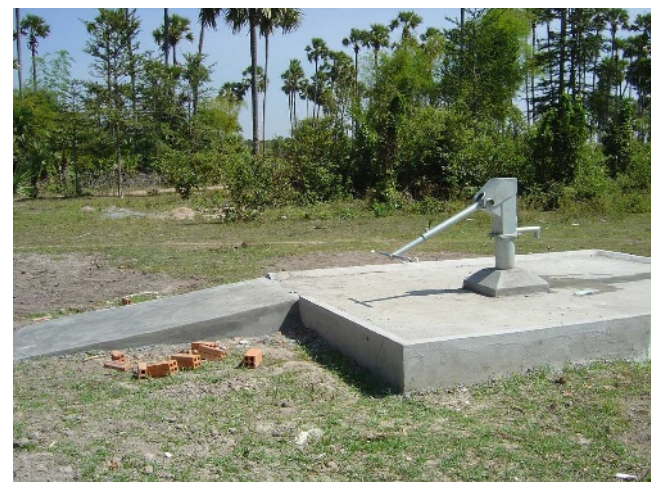
Figure 2. Handpump platform with ramp in Cambodia
