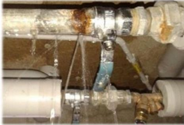
Figure 2.1 Water leakage in the buildings hot water system
